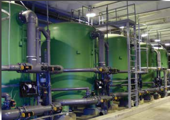
Industrial Process Water Treatment
