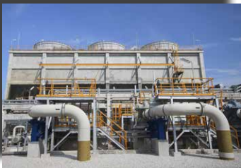
HVAC & Cooling Water Treatment
